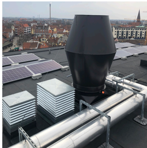
Air outlet from the kitchen
